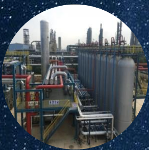
PSA提纯氢气技术 PSA purification hydrogen technology
