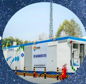
加氢站 Hydrogen refueling station
