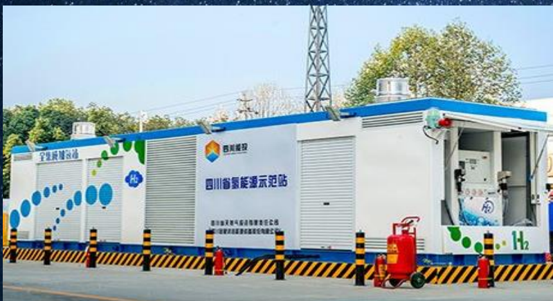
加氢站现场 Hydrogen station
